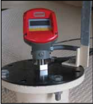
Actual installation on rice bin.
