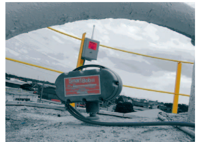
Cable-based system using a wireless transceiver at a cement block manufacturer.
