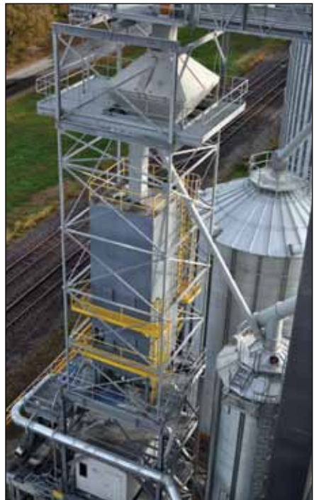
Overhead view of a 40,000-bph Intersystems gravity screener and 40,000-bph Compu-Weigh bulk weigh loadout scale.
