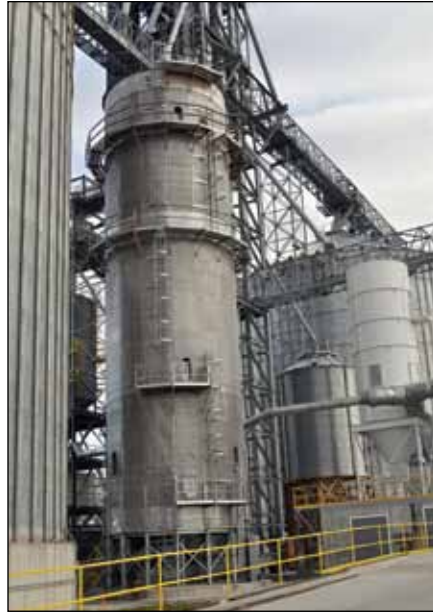
New natural-gas-fired 5,000-bph Zimmerman tower dryer in foreground and AIRLAN-CO baghouse dust control system to the rear.
